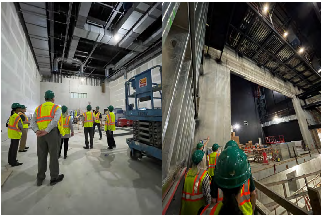
New Studio Theatre Black Box space under construction Hard hat tour of main theatre space in Hilberry Gateway
